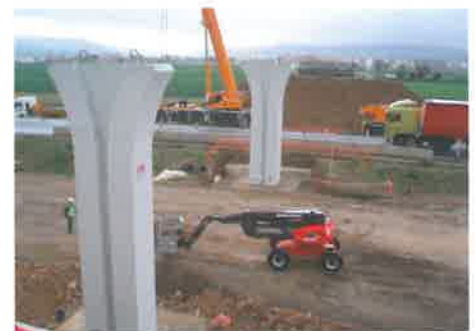
A-12 Highway (Camino de Santiago Highway) Hervias-Grañon section (La Rioja - SPAIN) Deck supported by palm shaped precast piers
