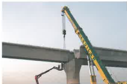
High Speed Train Viaduct - Section Mocejón - Toledo (SPAIN) Spans length: 36 m - 2 narrow TA-260 beams per span
