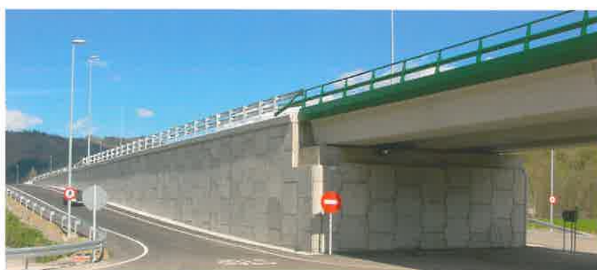
Pass under Corredor del Nalón road. Sotrandia - Barredas section (ASTURIAS - SPAIN) Reinforced earth abutment, supporting U beams
