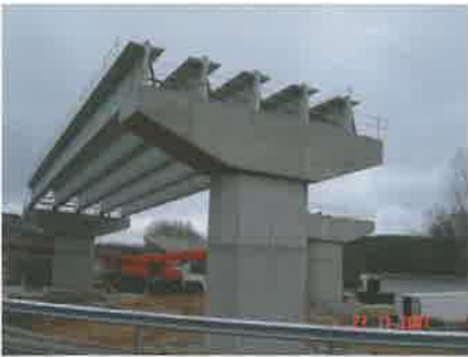
A-67 Highway (Palencia - SPAIN) - Section: Alar del Rey – Puebla de San Vicente - Viaduct 2.9 Solution: 5 IP-200 beams per span
