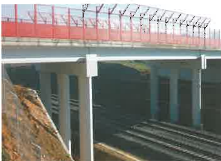
M-224 Road - Structure over high speed line railway in Torres de la Alameda (Madrid) 3 span deck, 4 IP-130 beams per span, supported by a portico, made up of 3 octagonal piers (9 m high) plus a lintel
