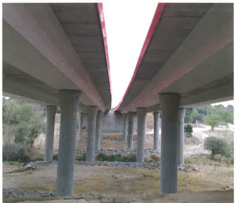
M-503 Highway - Viaduct over Aulencia river (Madrid - SPAIN) - 2 narrow TA-110 beams per span, supported by circular piers
