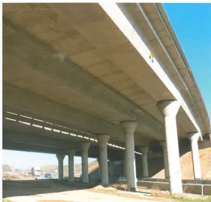
M-203 Highway - Viaduct over M-206 road (Madrid) - 3 narrow beams (1.50 m high) per span, supported by circular piers
