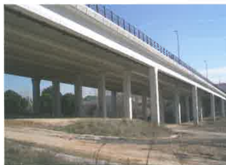
Viaduct over the Combos river, in Arroyomolinos (Madrid - SPAIN) 6 span deck, 6 IP-165 beams per span, supported by square piers (9 m high) with bell capital, without lintel
