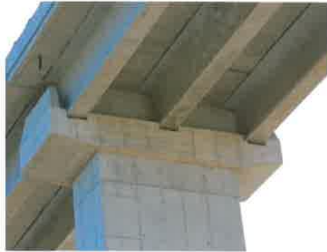
Seismic diaphragms between I beams to impede transversal movement and deck offset
